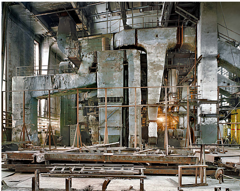
[Fig. 2] Erich Mendelsohn. Fábrica Red Banner, Central eléctrica (St. Petersburg, 1925-37) © Richard Pare.
